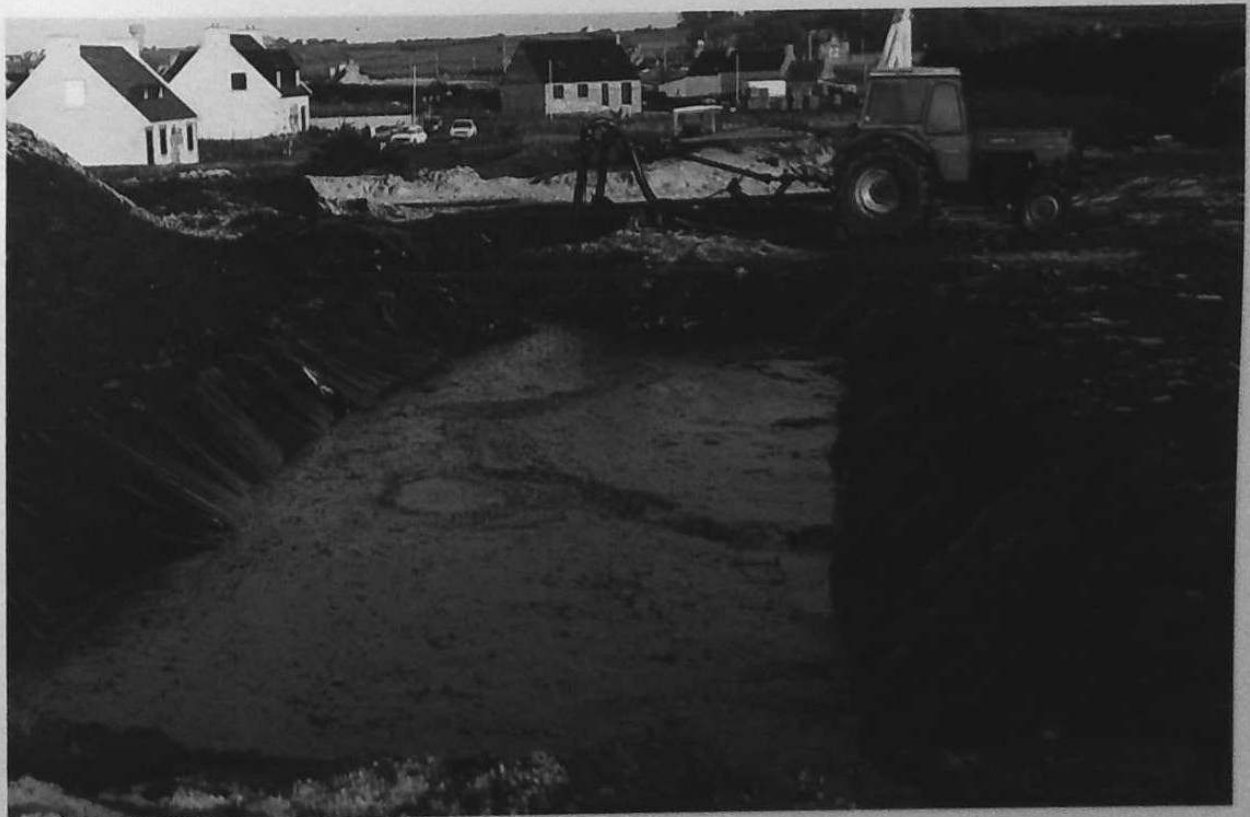
6-18. Close-up of the separation pits shown in Fig. 6-17. Note the use of dual pits with a screen between to separate the seaweed from the mousse.
