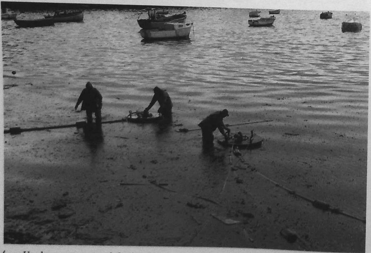
6-4. Workmen remove debris from two Acme skimmers which were among the very few to be used to skim the oil from the water and pump it into tank or vacuum trucks.
