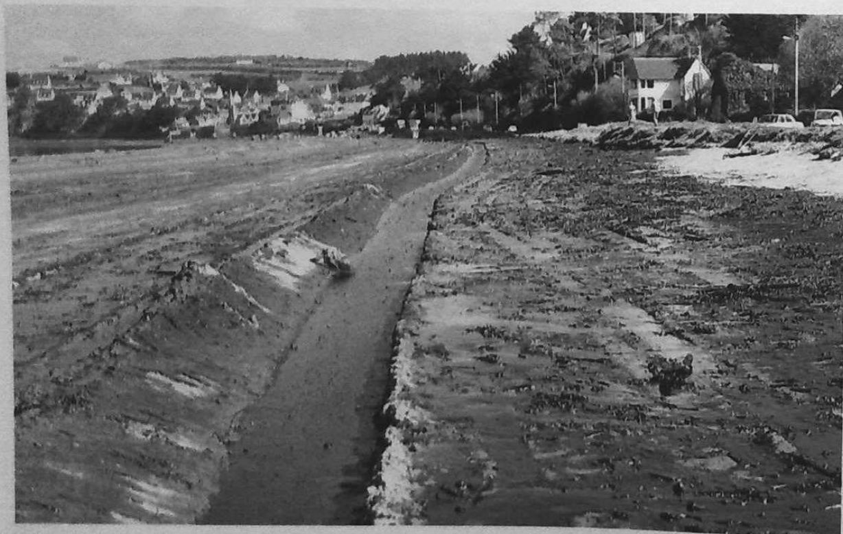
6-8. Trenches on the beach at St. Michel-en-Greve. The trenches proved effective in collecting the oil except where the sand surface was heavily marked with vehicle tracks.
