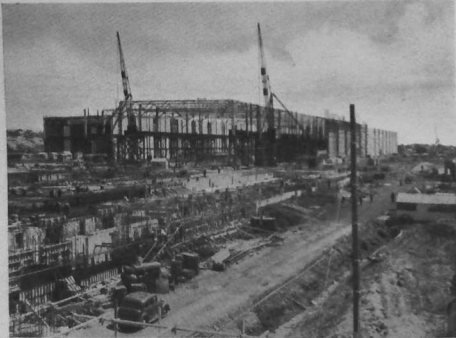
New Cold Reduction Plant, Llanelly, for the Steel Company of Wales Ltd.
